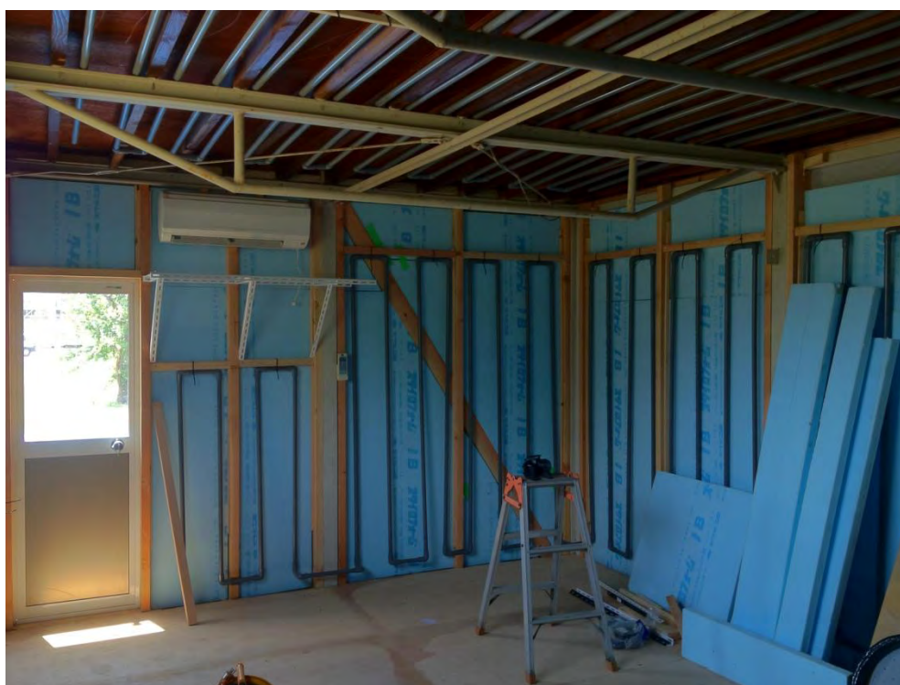
A 56—Piping network of the room at the study site on Tsushima campus, Okayama University (2).
