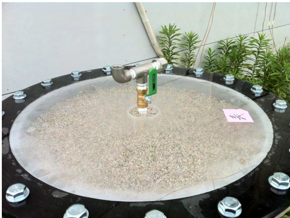
A 52—Picture of the charcoal filter at the field site showing the top with the fine gravel packed above the charcoal material, the lid and the connection for the pipe.
