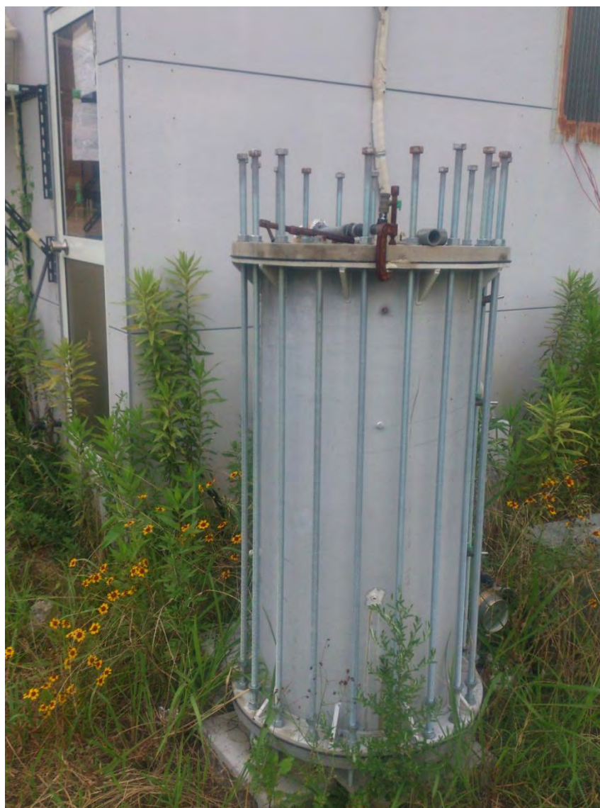
A 47—Charcoal filter column in front of the house at the study site on Tsushima campus, Okayama University.
