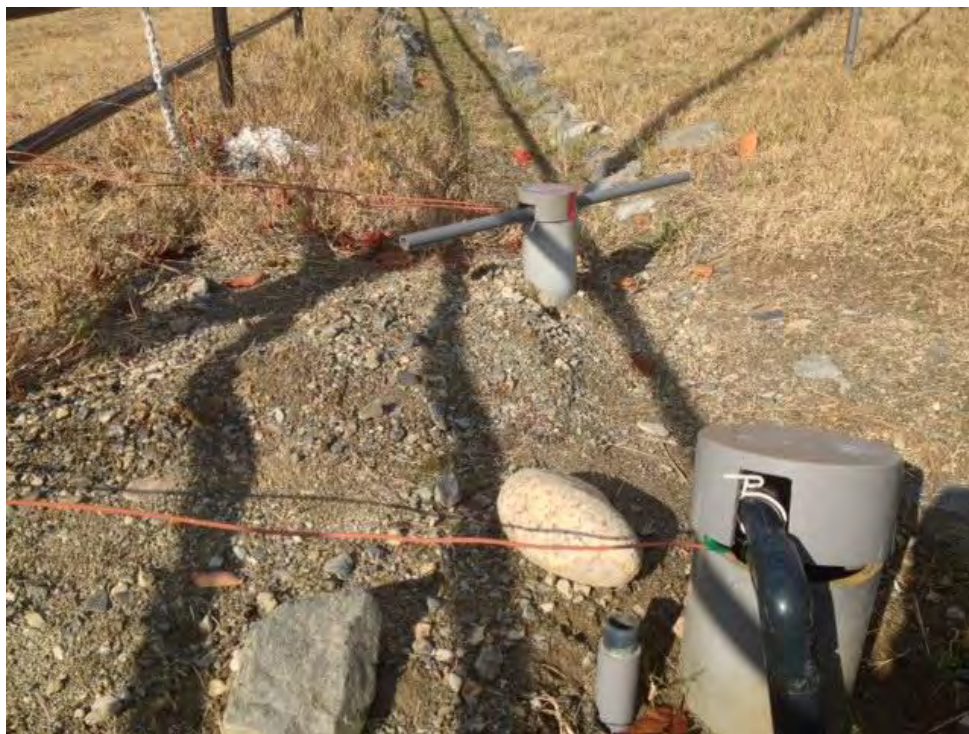
A 57—Set up of Temperature and head sensores in Injection well No. 1 (infront) and observation well No. 1’.
