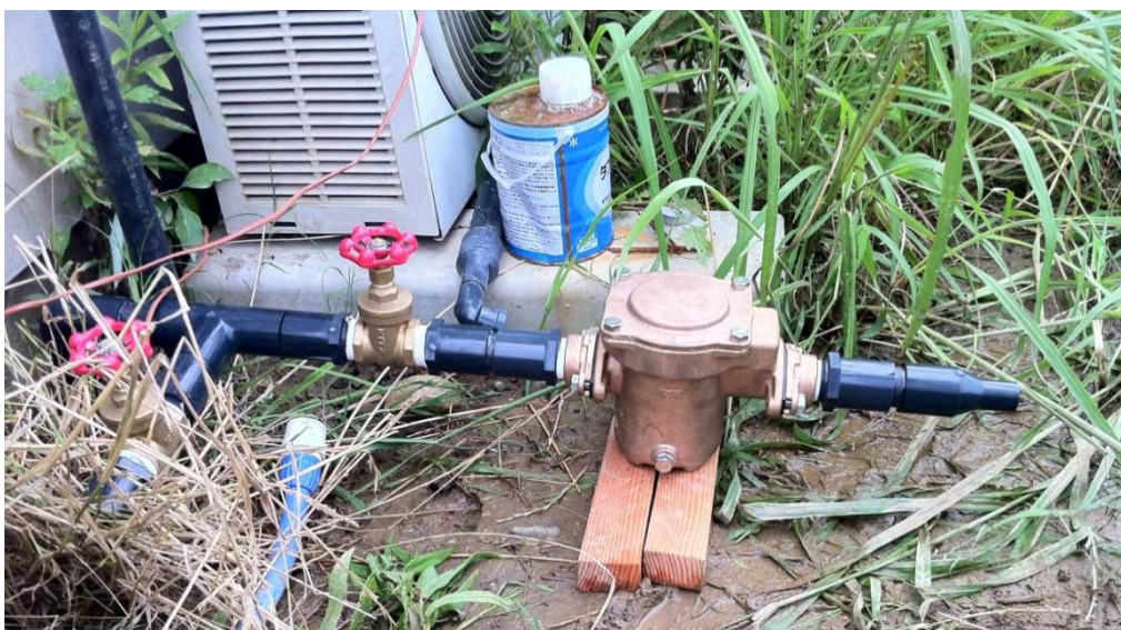
A 53—Small filter (100 mesh) installed HITACHI ® (GF-25V) before the charcoal filter in order to avoid clogging through fine particle and also to keep already build up iron flakes out of the filter inlet.
